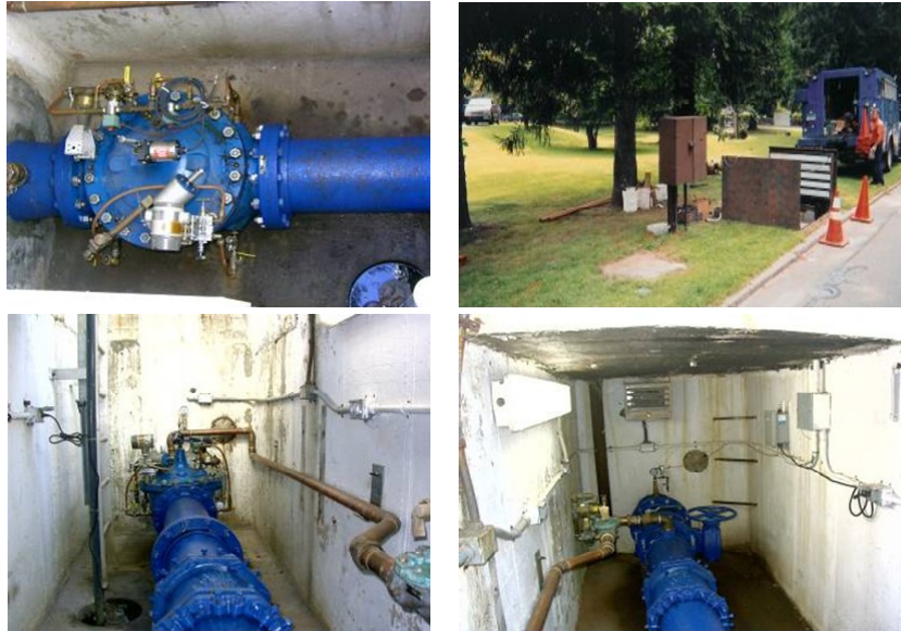
Stamford Pilot Program Site: 5' by 15' Vault with 8-inch Main and Claval PRV Located Next to Road with Electricity Available on nearby Utility Pole
