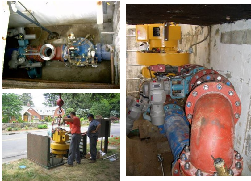
Stamford Pilot Program Site: Tee Flange installed Upstream of PRV Installed Flow-to-Wire Turbine, By-pass piping & electronic valves
