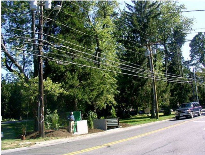
Stamford Pilot Program Site: Completed installation with 3 Single Phase Transformers, Underground Turbine, and Above Ground Control Panels
